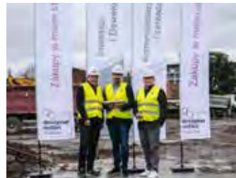
Inauguration of the construction works of Designer Outlet Kraków with representatives of KG Group and ROS Retail Outlet Shopping
